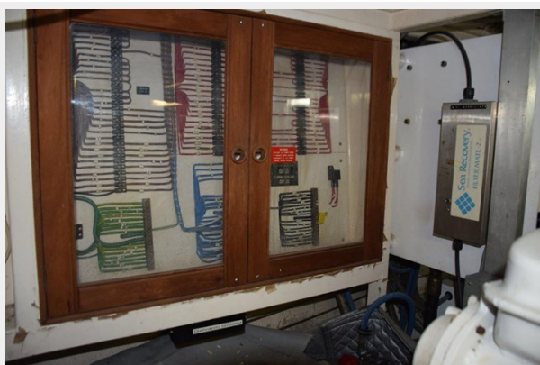
GB Wiring Cabinet
