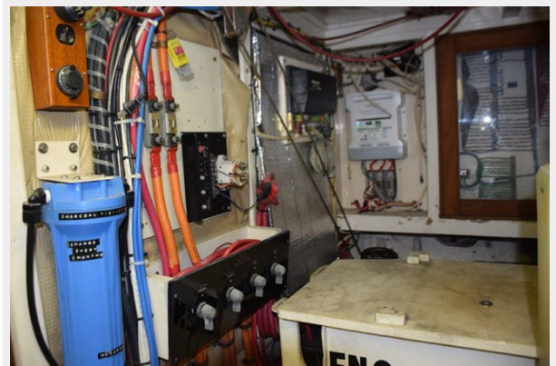
Forward Starboard Engine Room
