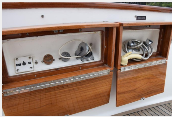
Aft Control for Glendinning Cablemaster, TV Phone Inlet Plugs, Freshwater Shower
