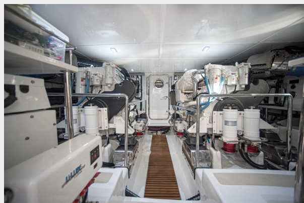
Engine Room facing Forward
