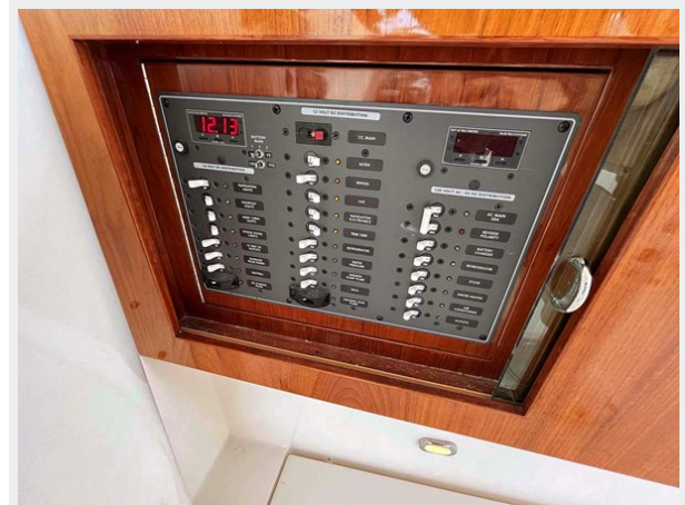
Electrical Panel at Helm
