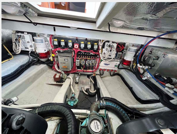
Engine Room Forward
