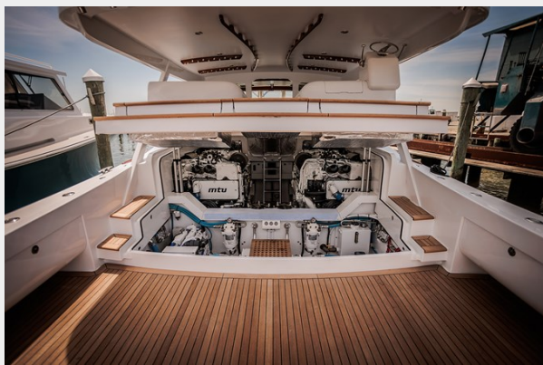
CY55 Engine Room
