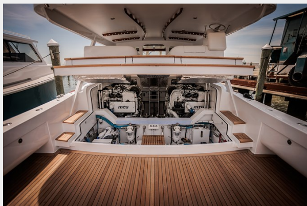
CY55 Engine Room
