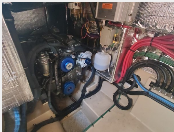
Harmony engine room
