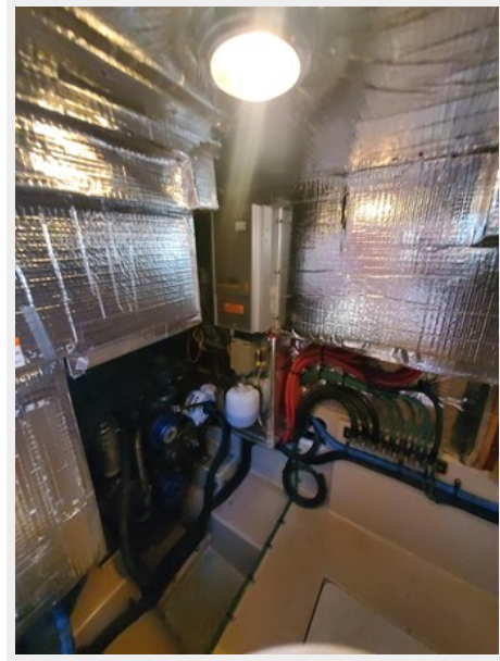
Harmony engine room
