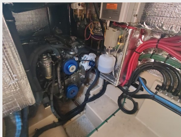
Harmony engine room
