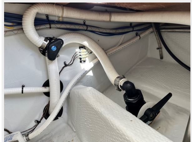
Holding Tank Y Valve
