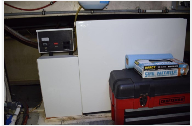
Onan Generator in Sound Shield
