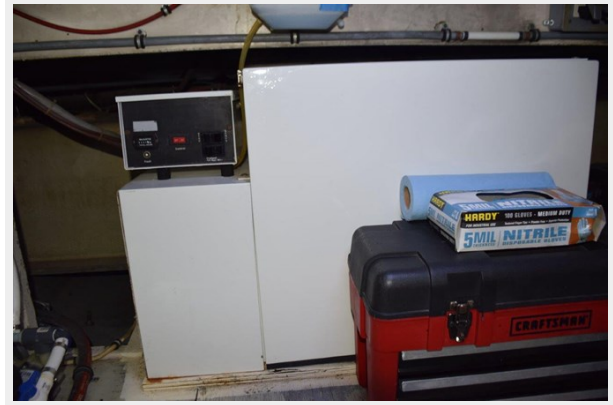
Onan Generator in Sound Shield
