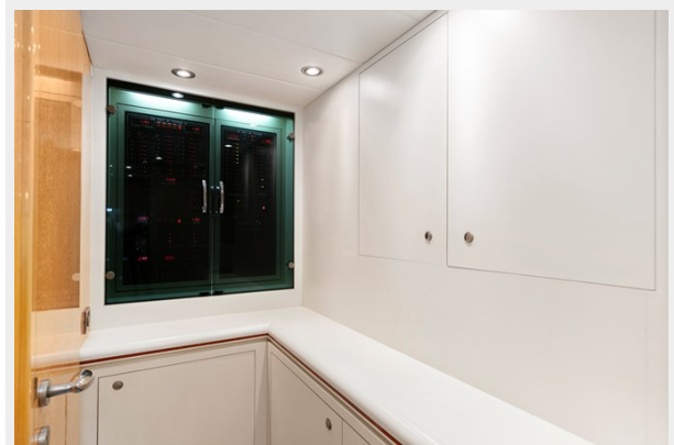
Electrical Distribution panel, crew area
