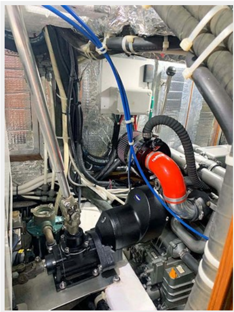
Engine Space Aft
