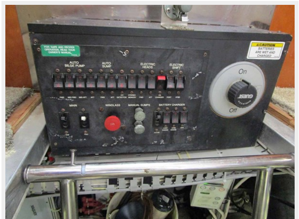
Engine room electrical panel
