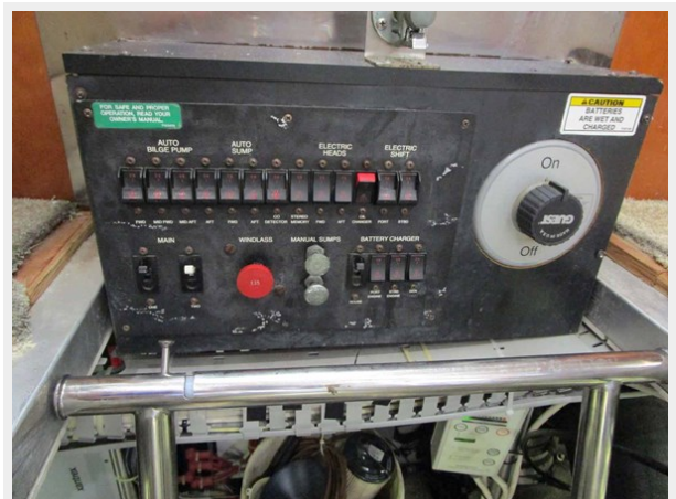
Engine room electrical panel
