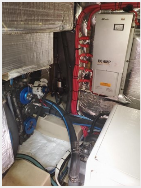
LadyM engine/genset wiring
