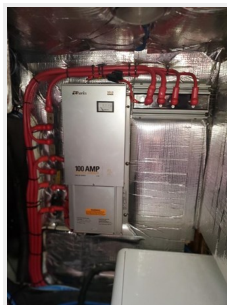
LadyM engine/genset room
