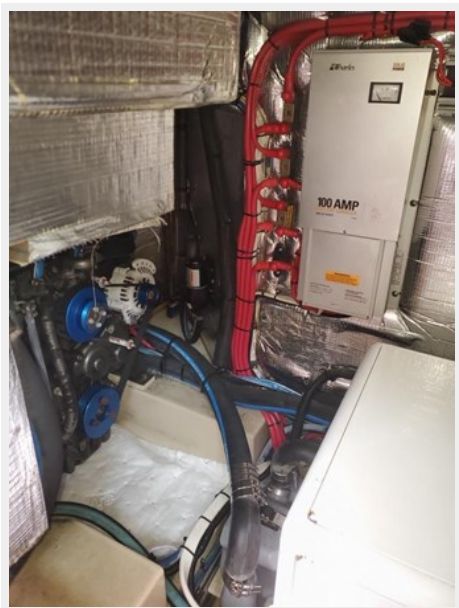
LadyM engine/genset wiring
