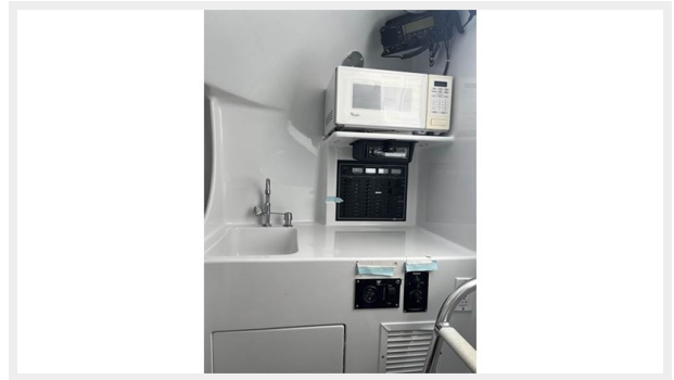
Microwave, Sink, Electrical Panel, A/C and Generator Controls
