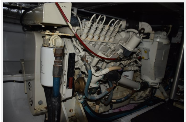
Starboard Cummins Diesel
