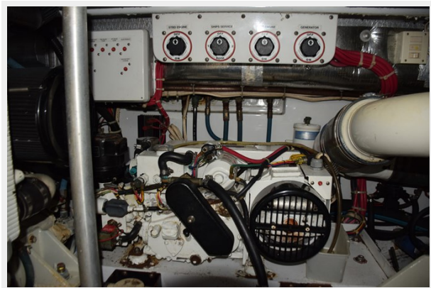
Battery Shutoff Switches and Parallel above Generator
