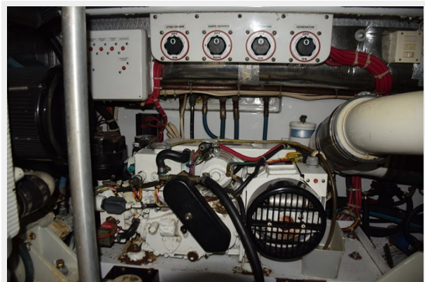
Battery Shutoff Switches and Parallel above Generator
