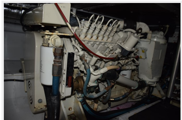
Starboard Cummins Diesel
