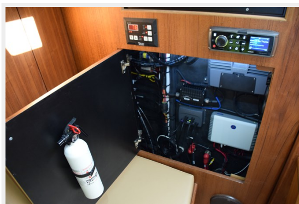
Organized Wiring and Electronics
