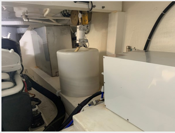
Engine Room Port
