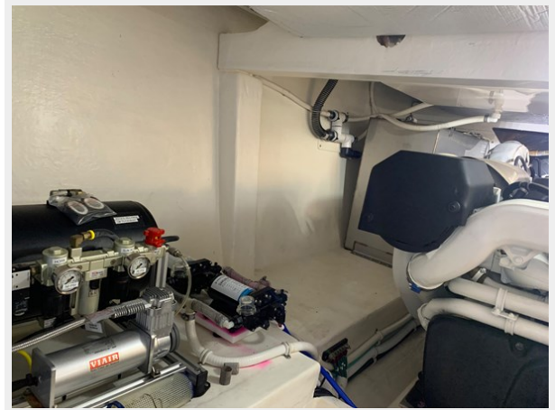
Engine Room Starboard
