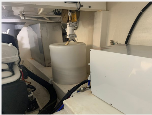
Engine Room Port
