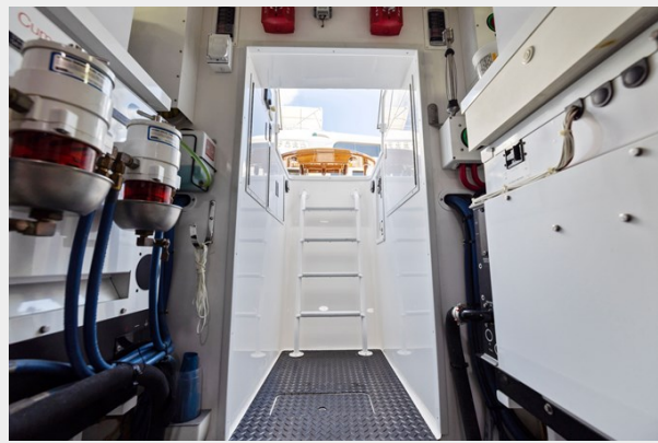
Entry to Engine Room
