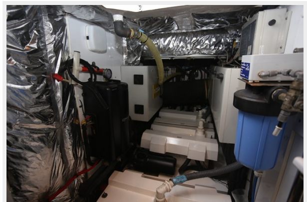
Princess 62 Engine Room
