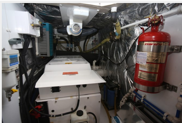
Princess 62 Engine Room
