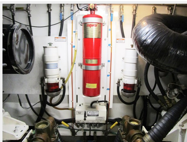
Center of Engine Room
