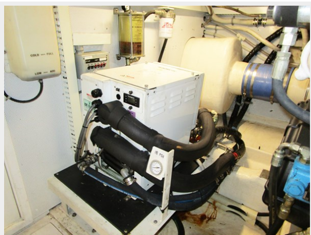
New A/C Chiller
