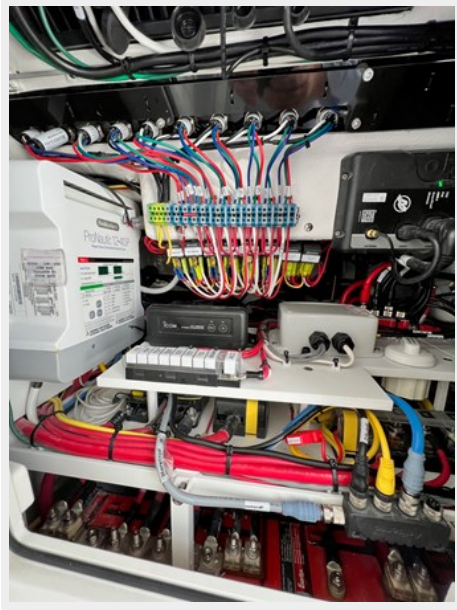
under console wiring
