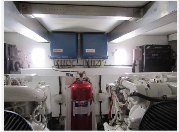
Engine Room Center
