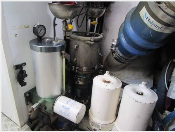
Aft of Port Engine
