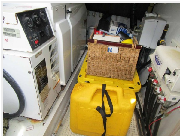
Generator in Lazarette
