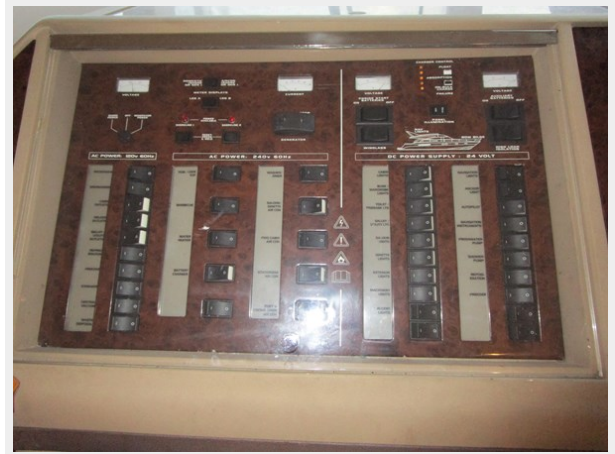
Main Electrical Panel
