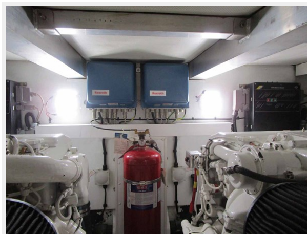
Engine Room Center
