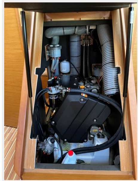
Engine Looking Aft
