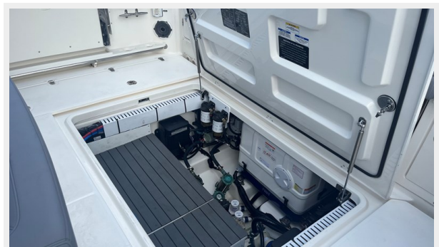
Generator and Aft Compartment
