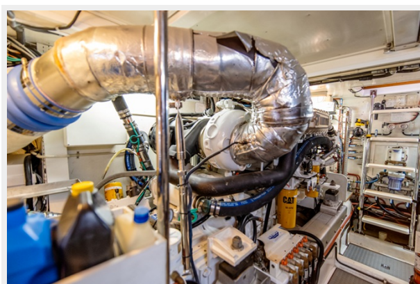
053 Engine Room SIERRA FOX 58_ Offshore
