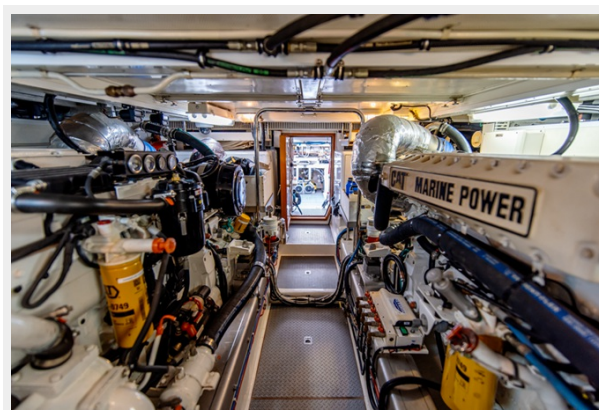
050 Engine Room SIERRA FOX 58_ Offshore
