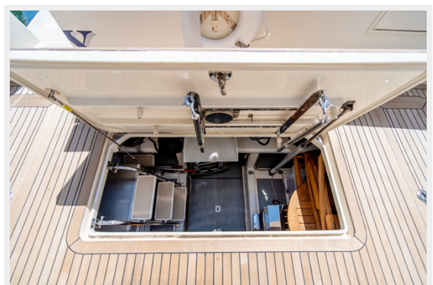
048 Engine Room SIERRA FOX 58_ Offshore
