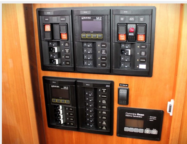
Main Electrical Panel
