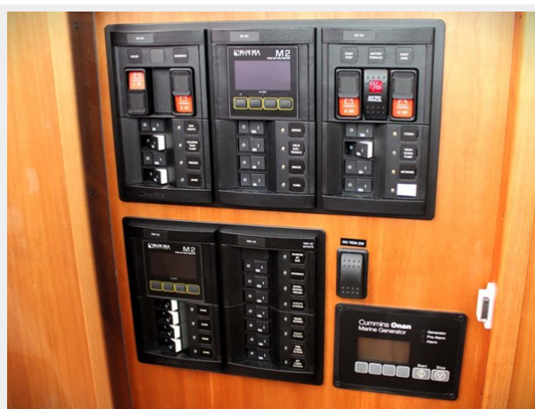
Main Electrical Panel
