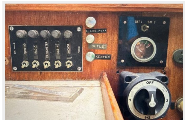
Electrical panel, gauges, & Master switch
