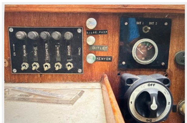
Electrical panel, gauges, & Master switch
