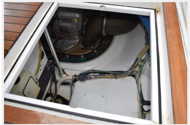
Aft Lazarette, Pod Access
