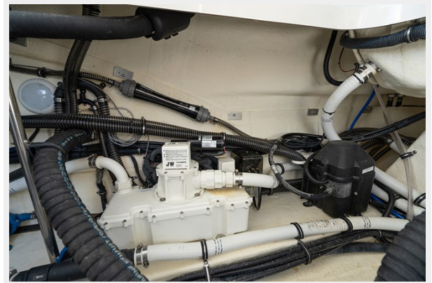
Engine room view 2
