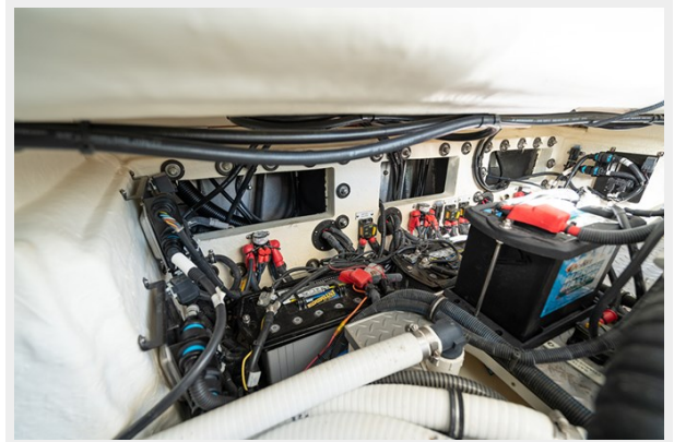
Engine room view 4
