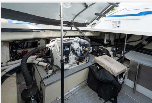
Engine room view 5
