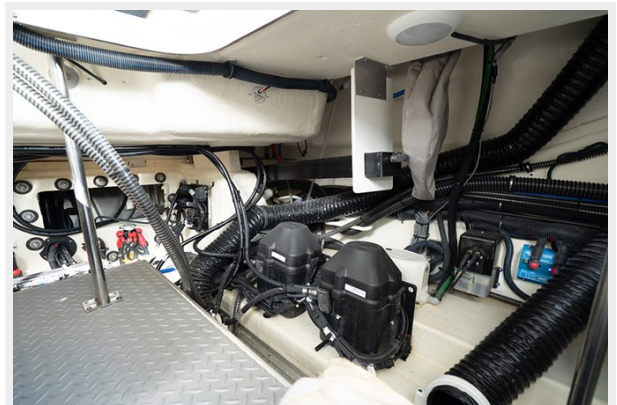
Engine room view 6
