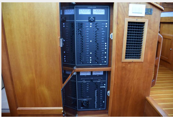
Main electrical panel
