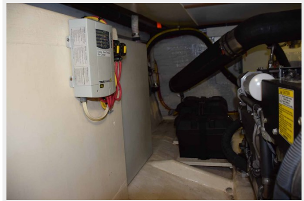
Battery charger and engine batteries
