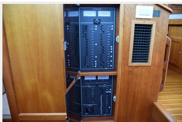
Main electrical panel
