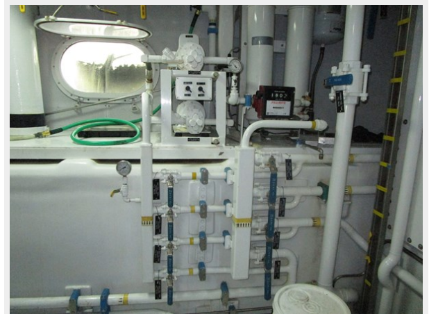
Fuel Transfer System
