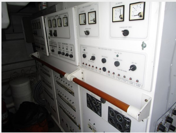
Lazarette Electric Panel
