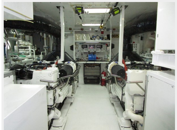
Engine Room Looking Forward
