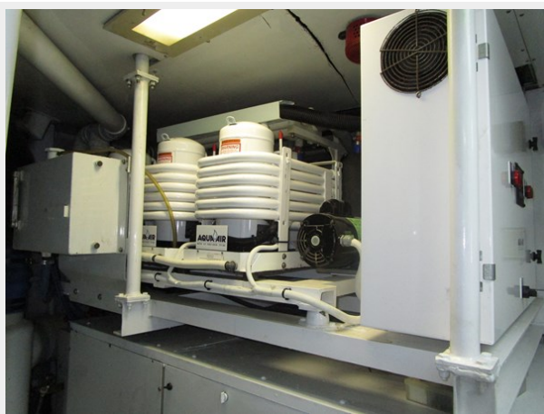
New A/C Plant
