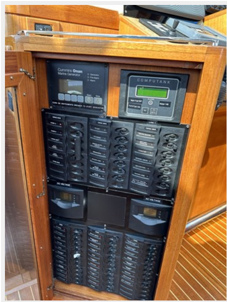
Main Electrical Panel
