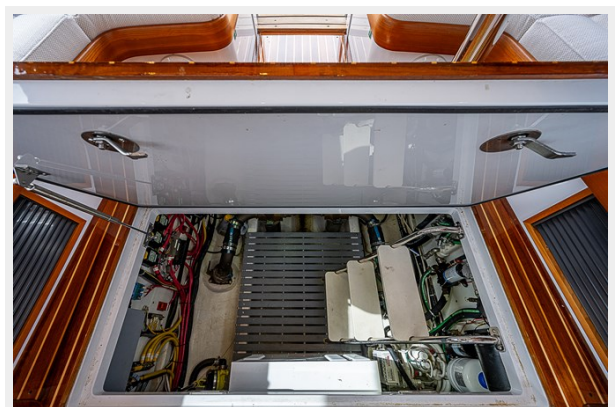
Engine Room Entrance
