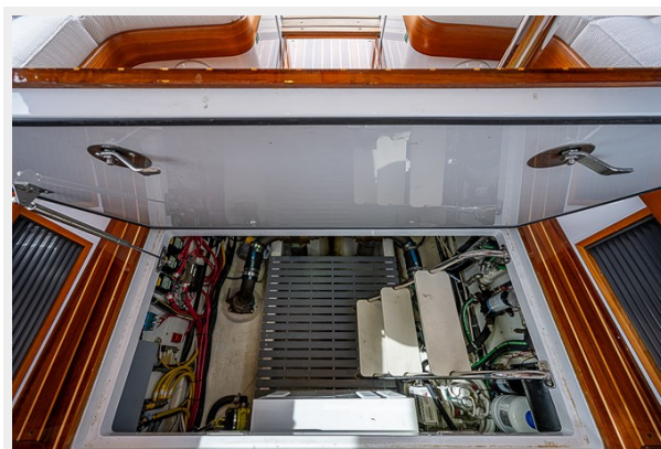
Engine Room Entrance
