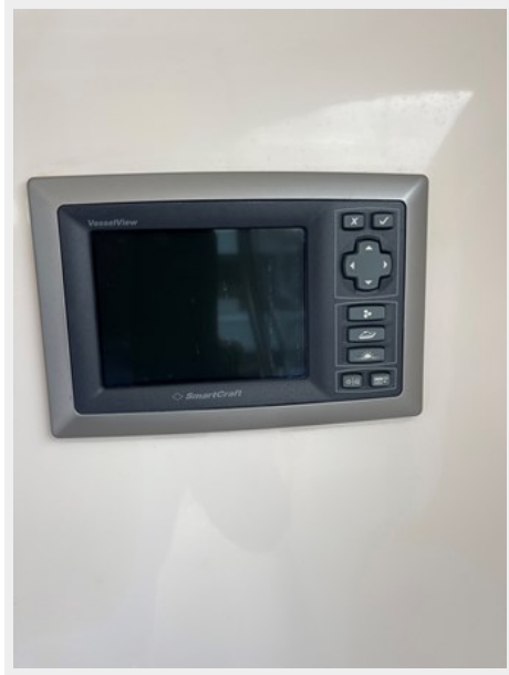
Aft Deck Engine Monitor
