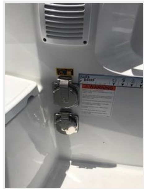
15 Shore power 30 amp
