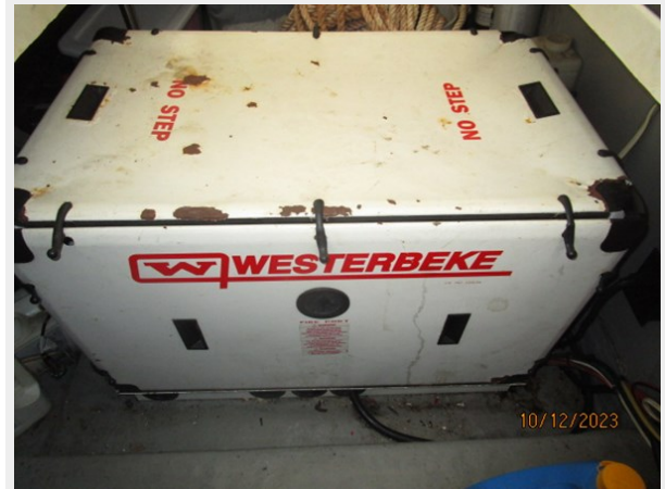
Pipe Dream generator soundbox 10-12-23
