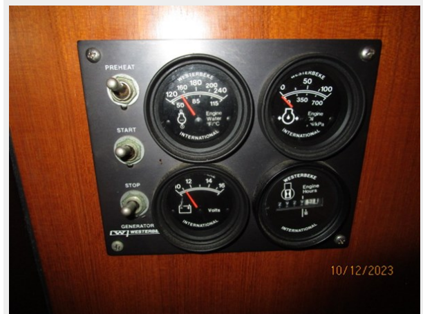
Pipe Dream generator panel 10-12-23
