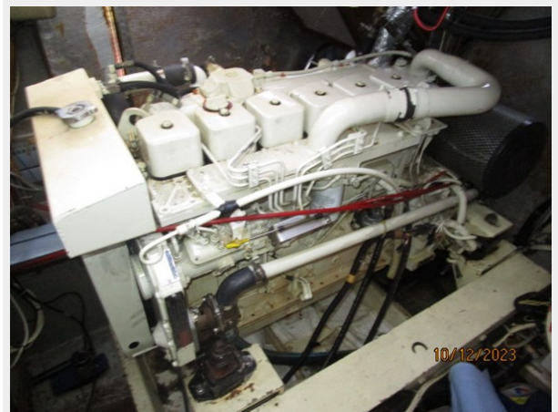
Pipe Dream main engine3 10-12-23
