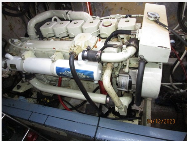
Pipe Dream main engine2 10-12-23
