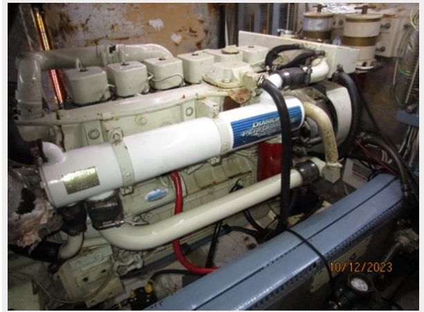
Pipe Dream main engine1 10-12-23
