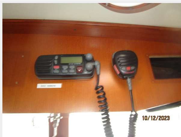
Pipe Dream pilothouse helm electronics1 10-12-23
