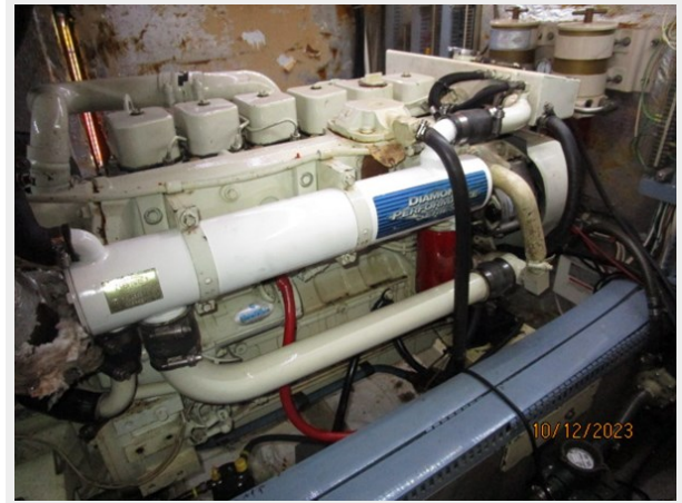
Pipe Dream main engine1 10-12-23
