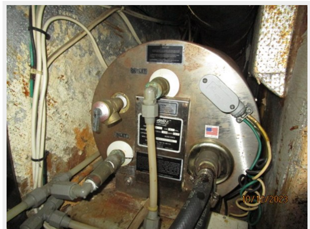
Pipe Dream water heater 10-12-23
