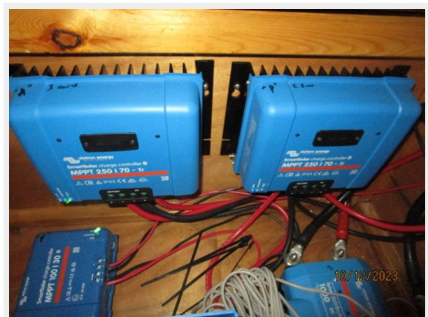
Pipe Dream solar controllers 10-12-23
