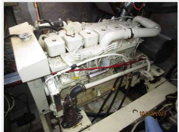
Pipe Dream main engine3 10-12-23
