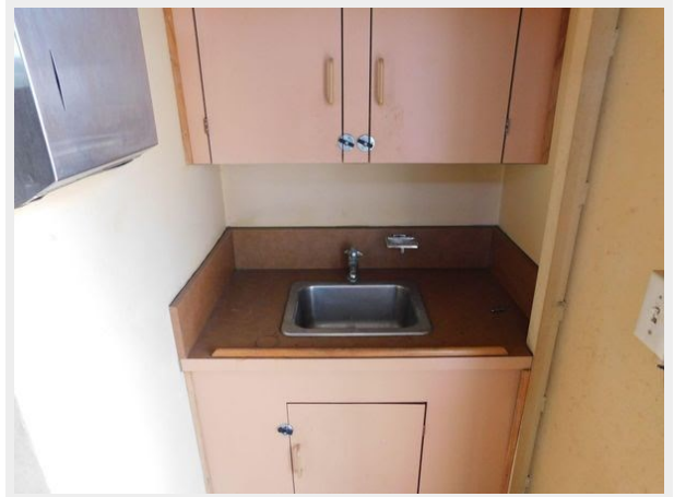
Commercial Fireboat - Galley
