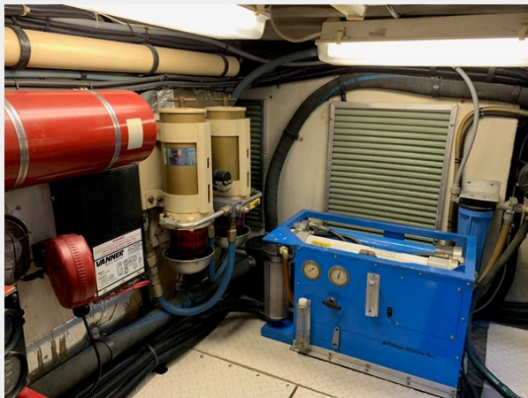
Engine Room Water Maker, Halon System, Racor
