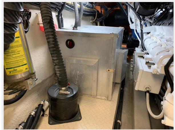
2nd Gen Set Engine Room
