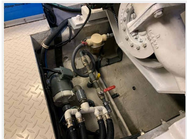
Engine Room Bilges
